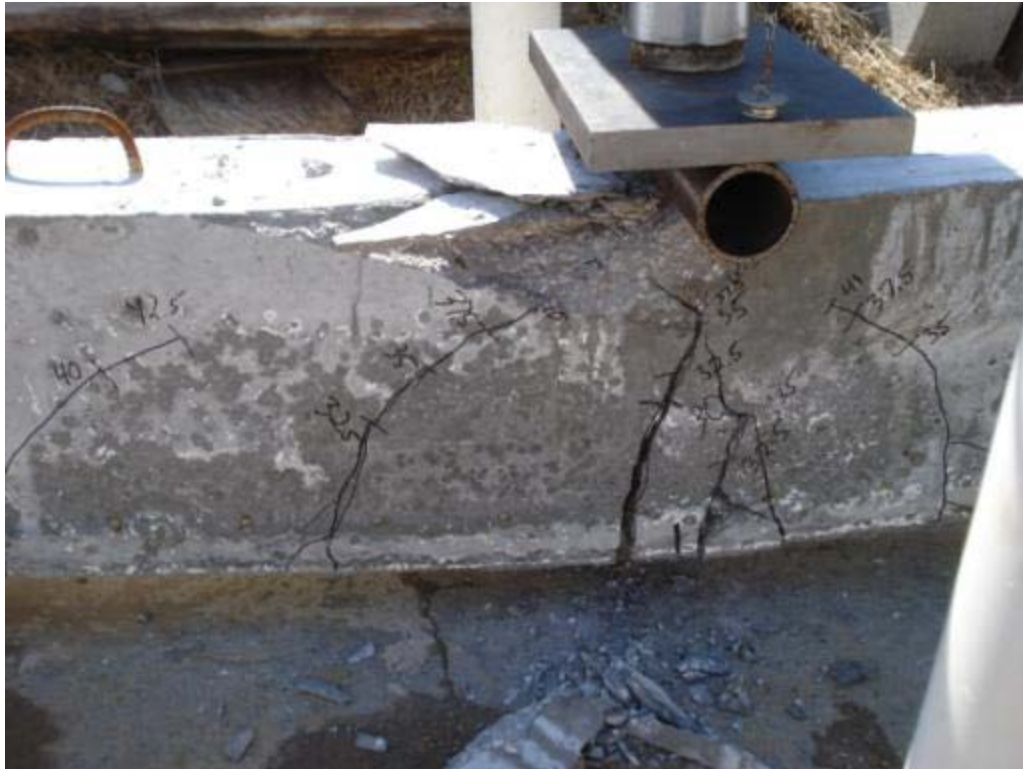
Figure 6.43: Cracking of specimen NSL-2L
