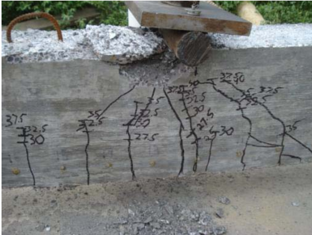
Figure 6.28: Failure of specimen NSS-3L
