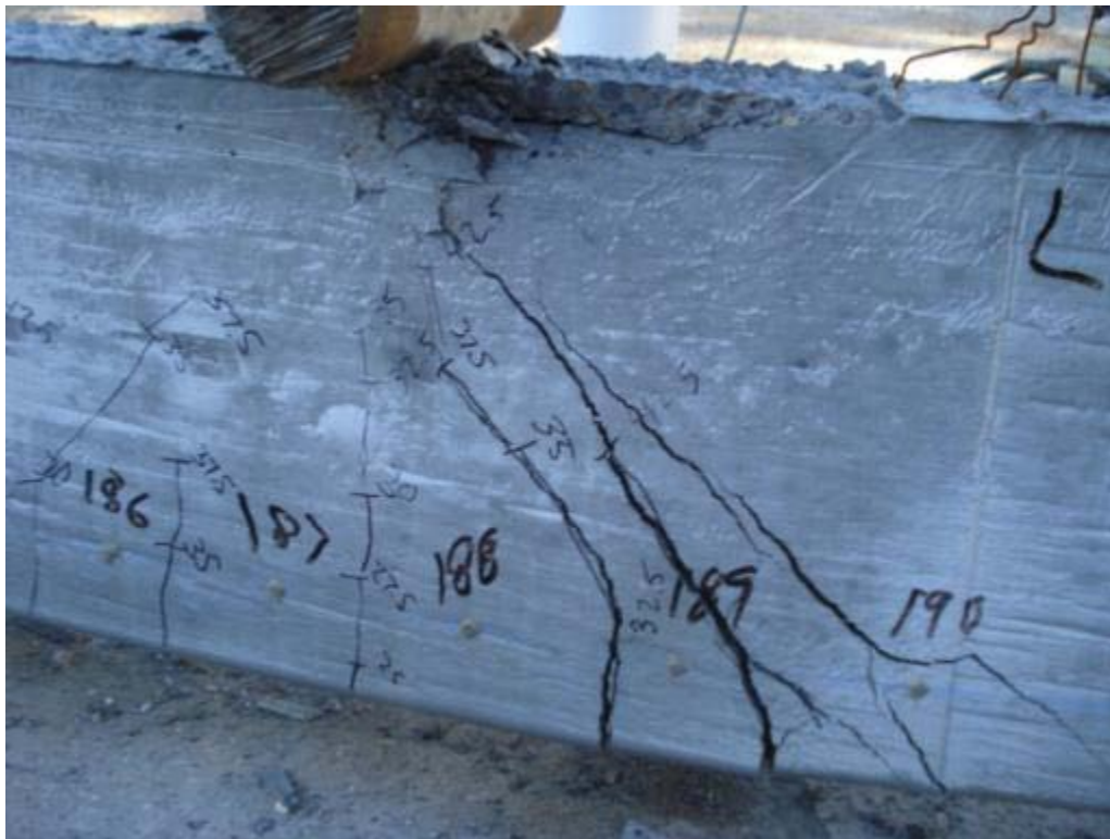
Figure 6.77: Cracking and failure of specimen HSS-3D showing crack width
