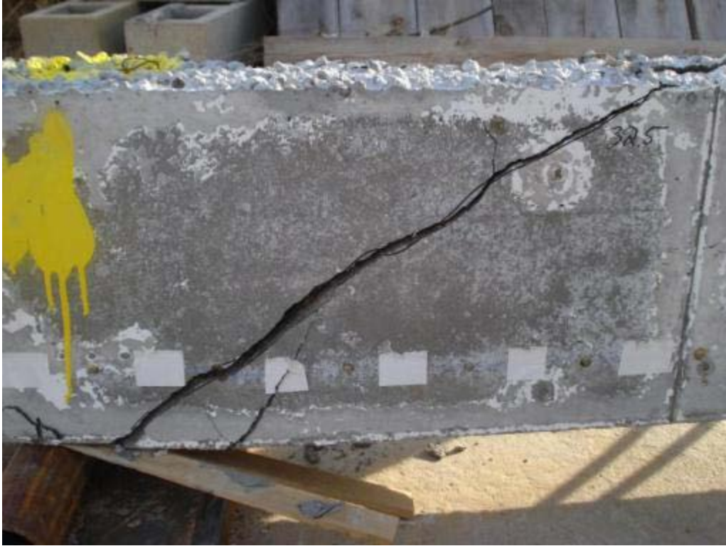
Figure 6.9: Shear cracking of specimen NSC-3D
