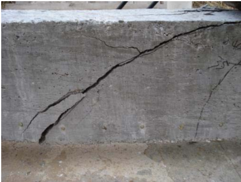
Figure 6.45: Shear cracking of specimen NSL-3D
