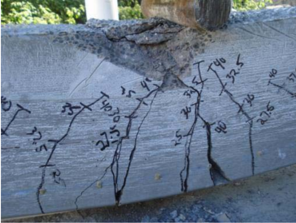
Figure 6.75: Cracking and failure of specimen HSS-2L showing crack width
