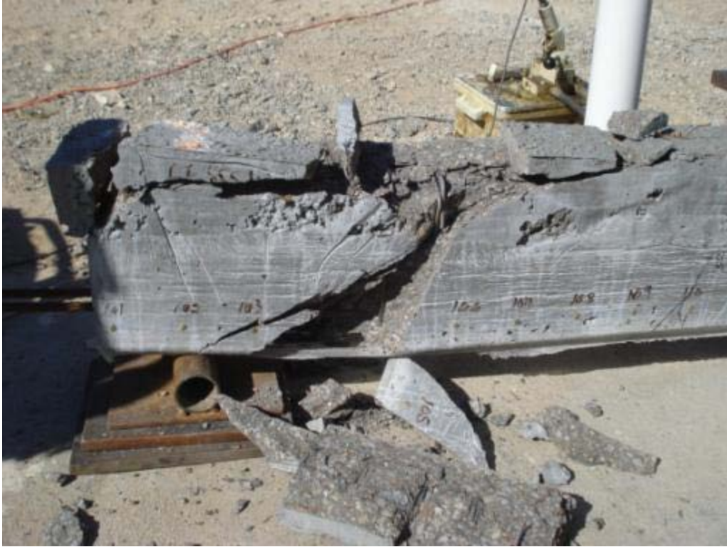
Figure 6.63: Shear failure of specimen HSC-3L
