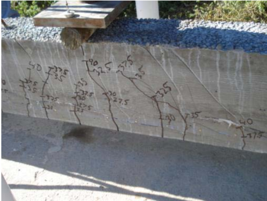
Figure 6.55: Cracking of specimen HSC-1L
